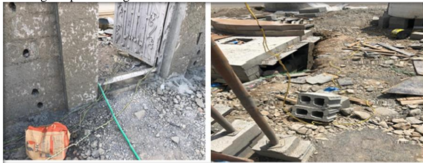
Figure 4. Bad electrical wiring and routing
