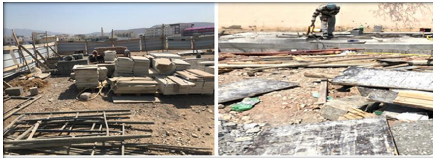
Figure 3. Poor flooring conditions
