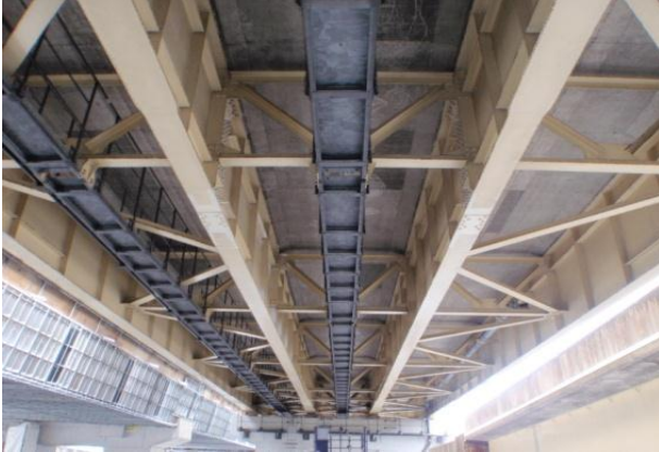
Figure 2. Condition of the target structure
