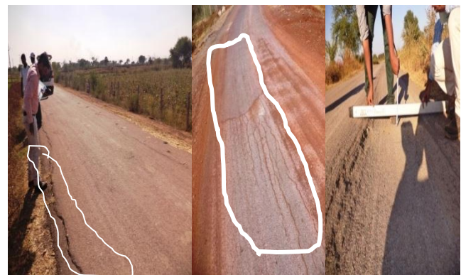
Plate 1: High severity Edge cracking
