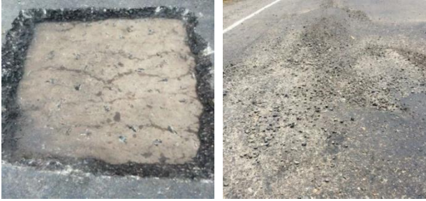
Figure 6. Cracks at Bottom 100mm Asphalt Layer Surface. Figure 7. Heaving of pavement surface
