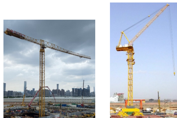
(a) Fixed type (b) Traveling type [10] Fig. 1. Tower crane types (classified by traveling mechanism).
