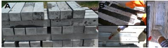
Figure 1. A) Concrete beam samples and B) Application of CFRP on the surface of reinforced concrete samples.
