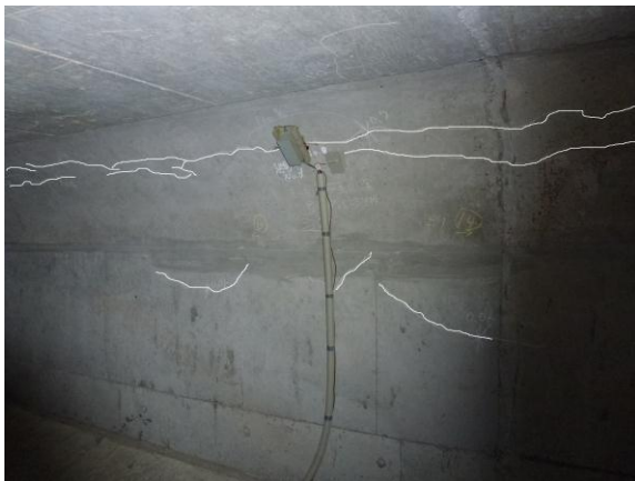
Figure 5. Cracks inside box girder
