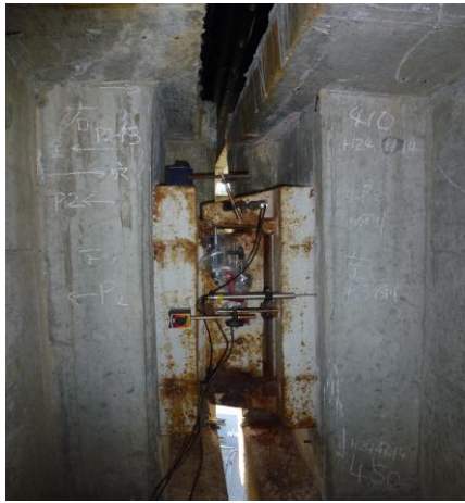
Figure 4. Joints's broken tracks
