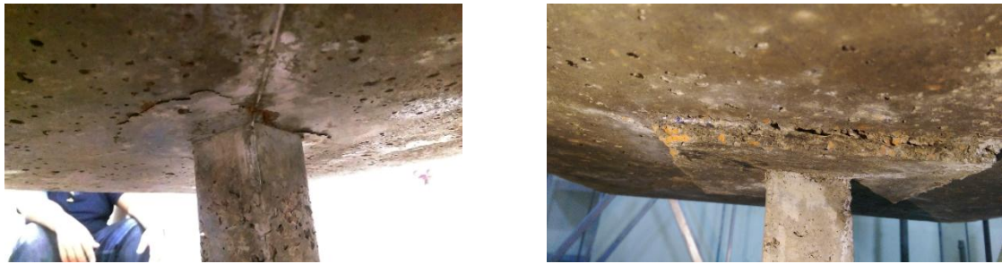
Figure 4. Damage behavior of M1-UR of concrete mix ratio of 1:2:4 after 25 sec dynamic test (left) and M2-UR of concrete mix ratio of 1:1.5:3 after 20 sec dynamic test (right).
