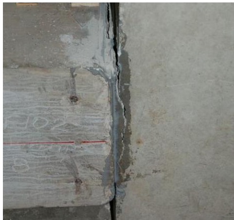
(b) Side view of the failed interface
