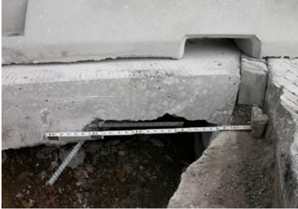
Figure 1. Paving notch failure/deterioration.
