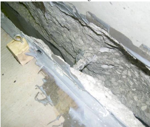
(b) Failed abutment concrete
