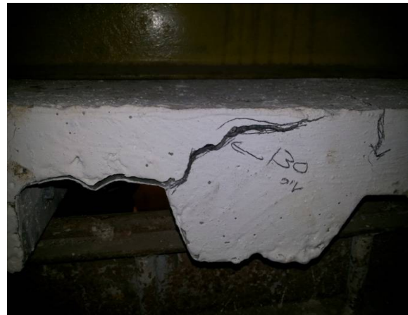
Figure 6: Vertical Separation and Diagonal Crack on CS
