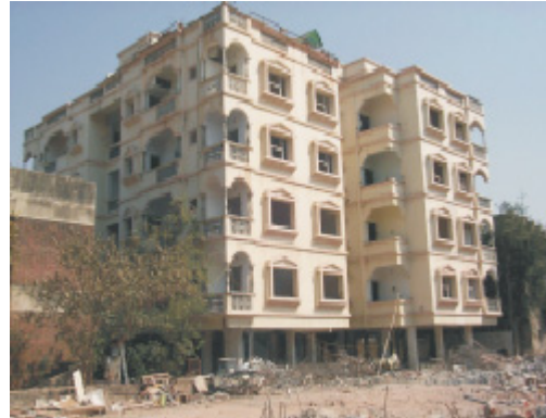
Figure 3: A Damaged Reinforced Concrete Frame Buildings With Open First Storey And Brick Masonry Infills
