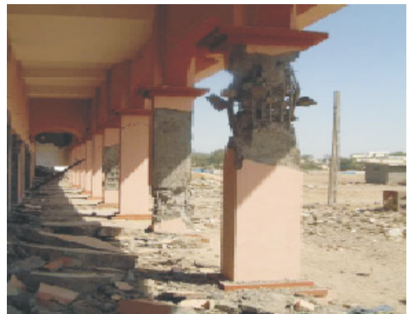
Figure 4: Failure of Column Through Plastic Hinge
