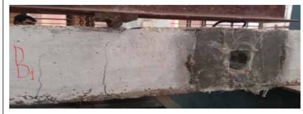
Figure 23: Cracking Pattern for Beam 1
