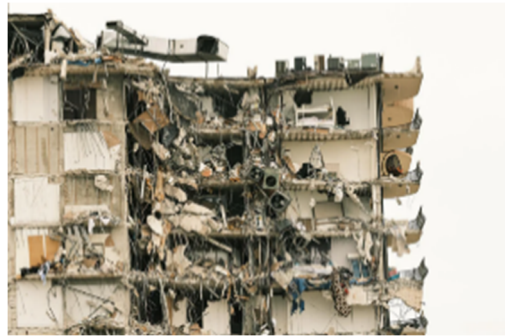
Fig. 9. Enlarged photo of a collapsed section.
