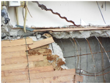
Fig. 10. Cross-section of a collapsed floor.
